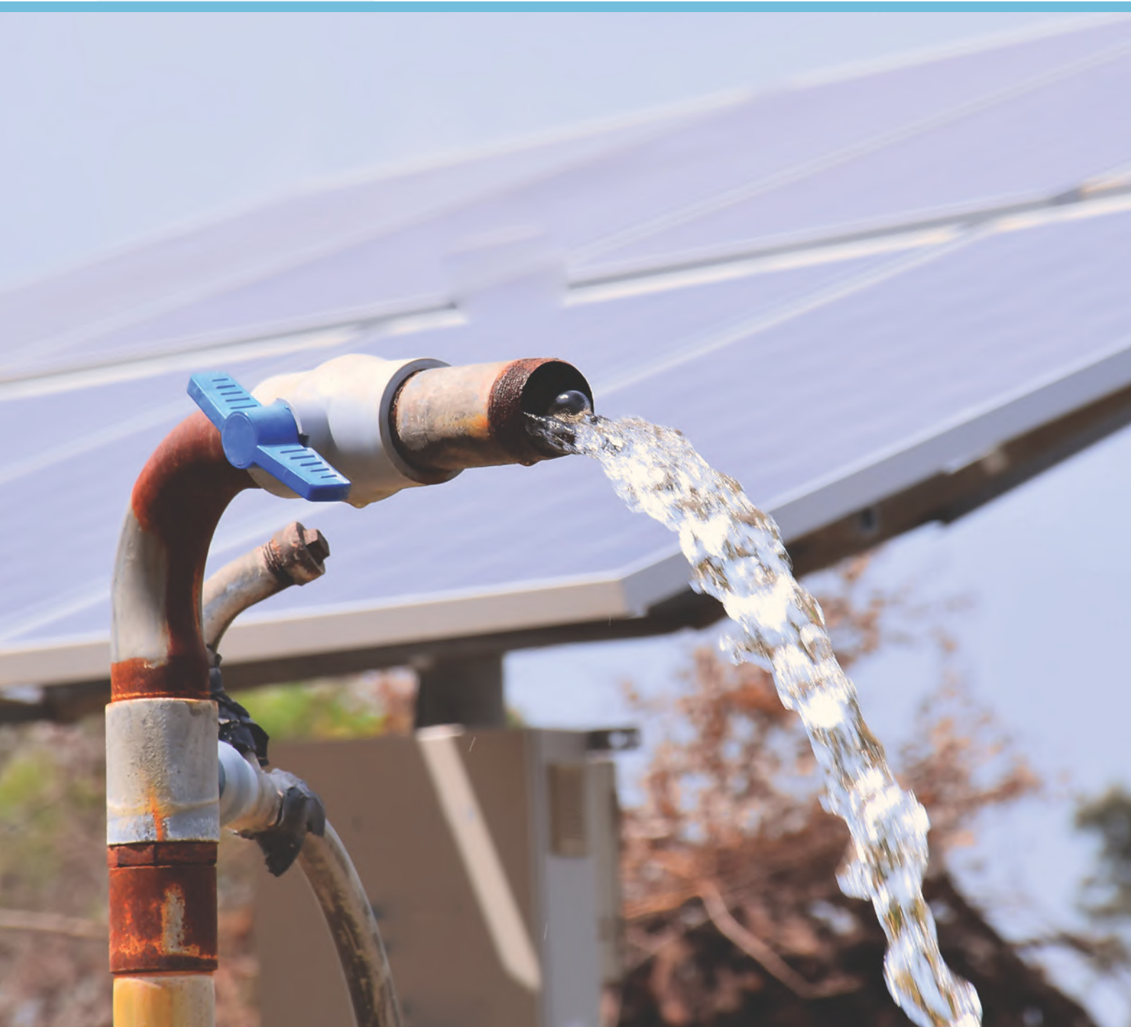
Equipment for a solar-based irrigation project.
