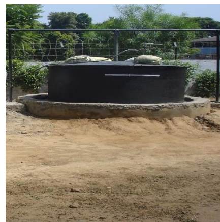
Figure 19: Paddy straw-based bio-gas plant
