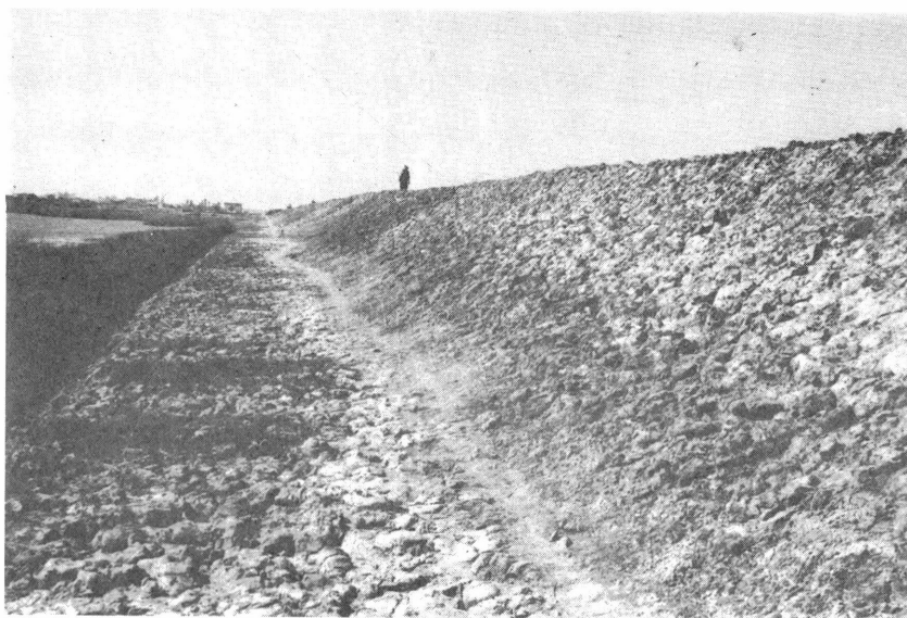
Figure 9. View of the land side of the dyke showing the 2 m wide berm.
