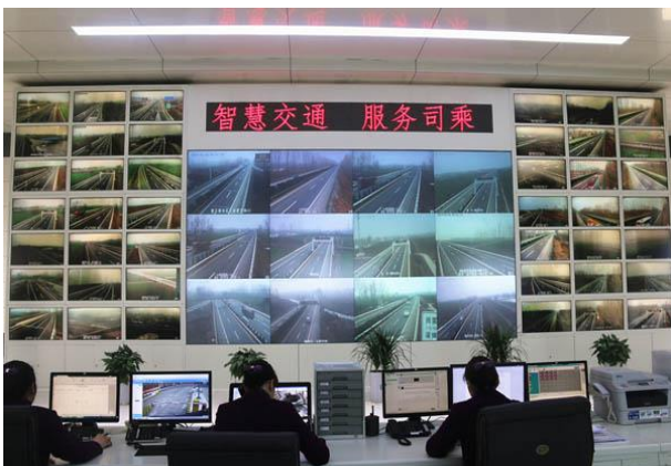
Figure 3. Control room of the Highway Monitoring and Management System in Anhui.
