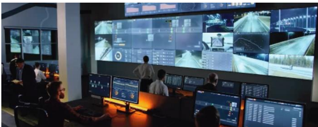
Figure 19. Interior view of the Central Ring Road's ITS control room.
