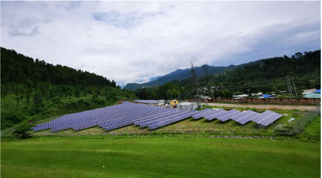
1.28 MWp Solar Plant developed under 25 MWp Grid Tied SolarFarm Project (Location_ nearby Devighat Hydropower Forebay Area) Commissionin Feb 2021
